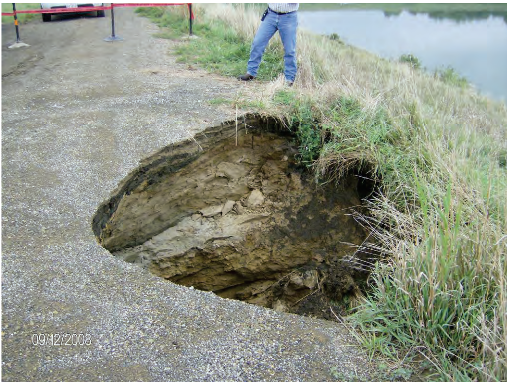
View of Sinkhole Looking Southeast Along Dike
