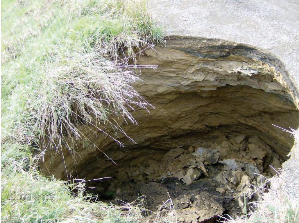
Close-Up of Sinkhole
