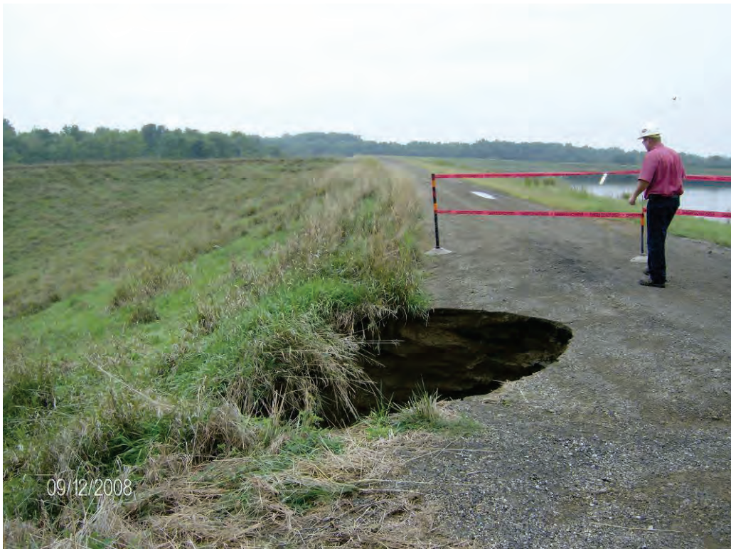
View of Sinkhole Looking Northwest Along Dike
