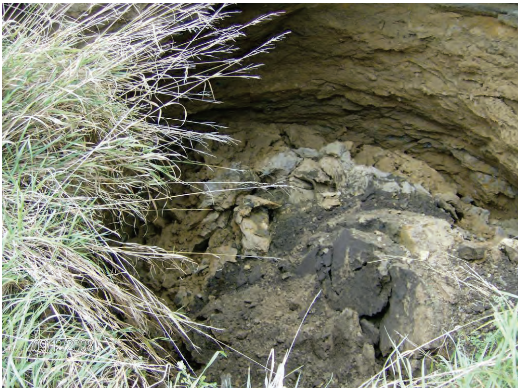
View of Bottom of Sinkhole
